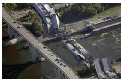
35W bridge collapse (2007)
