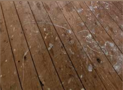
Chipped paint and signs of wear on the original wooden floor indicate long-term use and no recent renovation.
