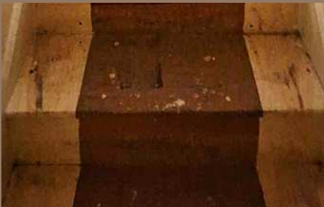
Worn wooden stair treads indicate heavy traffic and aging of the material.
